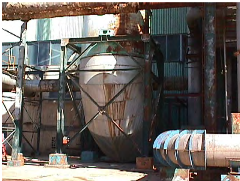
Figure 9. Corrosion of a carbon steel pipe under insulation.
