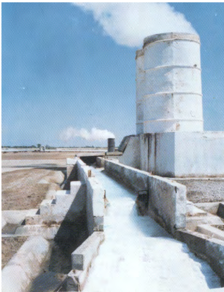
Figure 15. Corrosion in concrete structures used to separate steam from water and to operate steam silencers.
