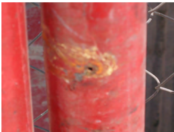
Figure 2. External pitting caused by biocorrosion on the internal surface of a carbon steel pipe in a fire extinguisher system.
