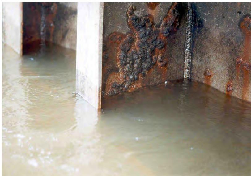
Figure 5. Corrosion on the gates dam on the Colorado River, Baja California, Mexico
