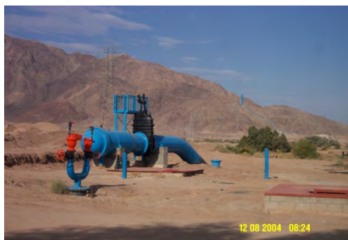
Figure 7. Valve system of a desert water aqueduct.
